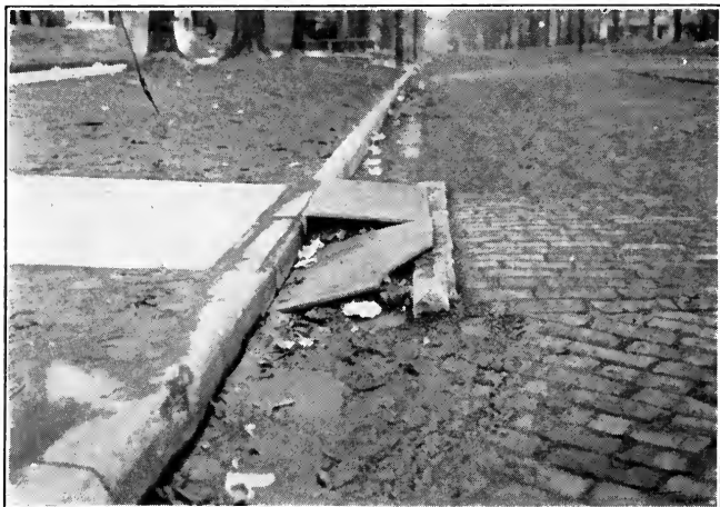
A DANGEROUS CONDITION AT A GUTTER CROSSING The need for improvement extends further, as seen by the condition of the gutter.
